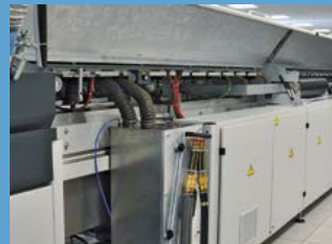
Maintenance on the fly: machine is operating while the condensation management is being cleaned
